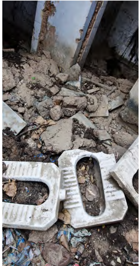
A derelict toilet facility at Ghazipur, Delhi
